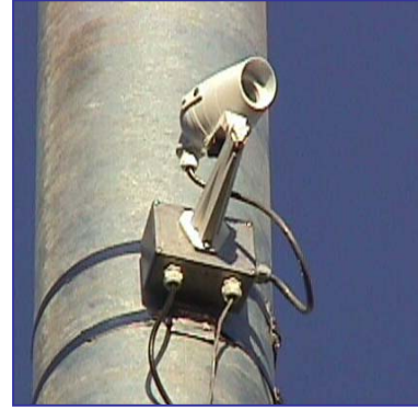
CAM Junction Box w/ mounted EX-10
